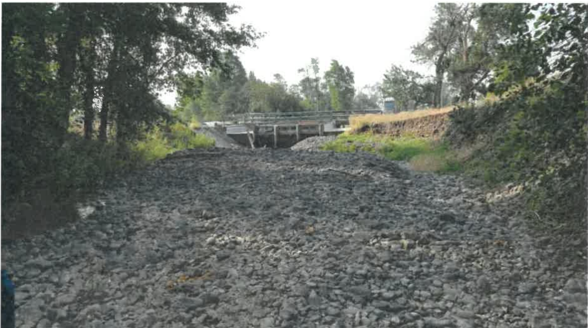
Photo 2: View downstream to KRD intake structure. Note perched bedload elevation is higher than the KRD structure.
