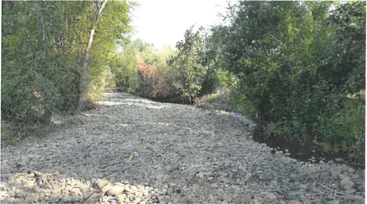
Photo 1. Accumulated sediment upstream of the KRD canal intake has forced Naneum Creek out of the current channel. Naneum Creek flows are seen on the right edge of the photo. Keeping flows isolated like this will allow a dry work area for equipment.
