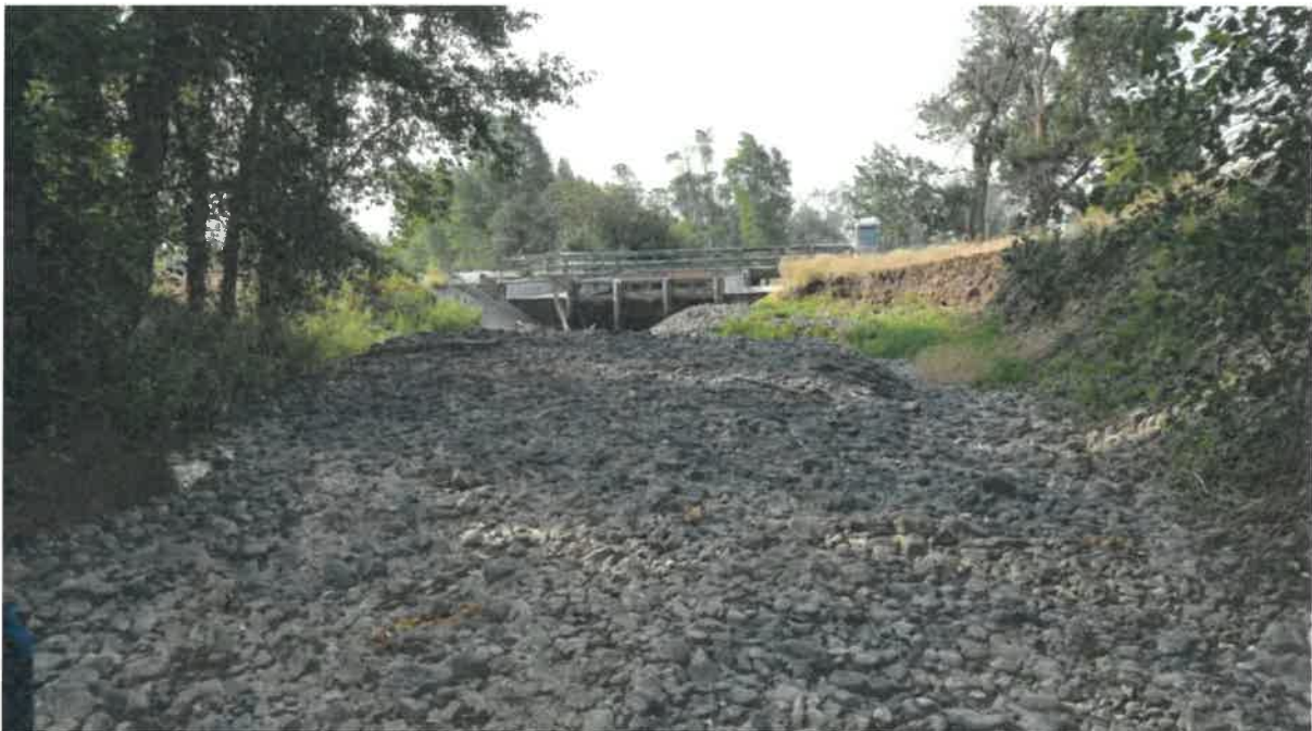
Photo 2: View downstream to KRD intake structure. Note perched bedload elevation is higher than the KRD structure.
