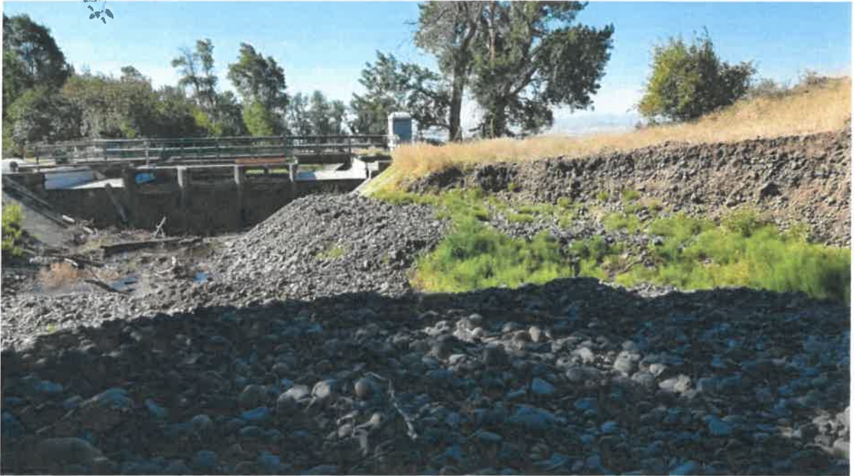
Photo 3. Eroded bank just upstream of the KRD canal intake structure that requires armoring. Sediment deposition in the channel forced the creek into this bank, causing rapid erosion.
